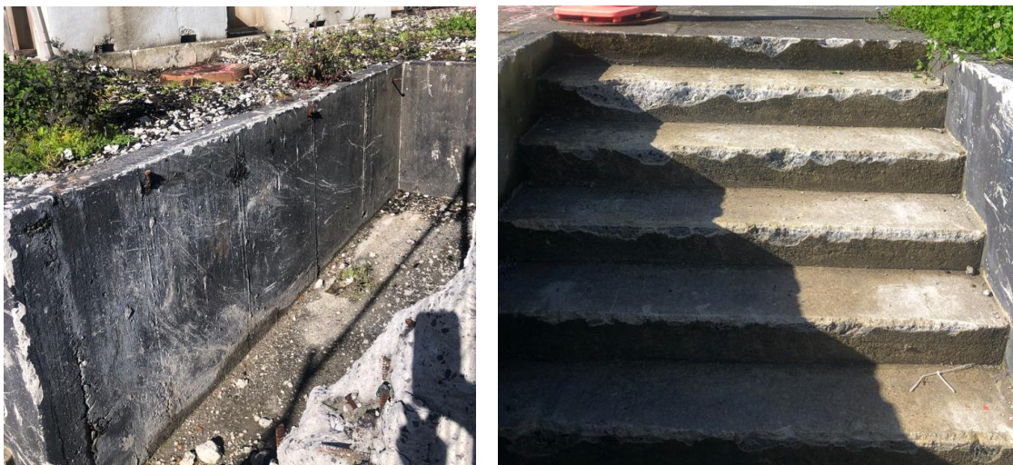
Figure 26. Left photograph showing a concrete retaining wall, and right photograph showing a set of concrete steps, both cut into the southern part of the Project Area
